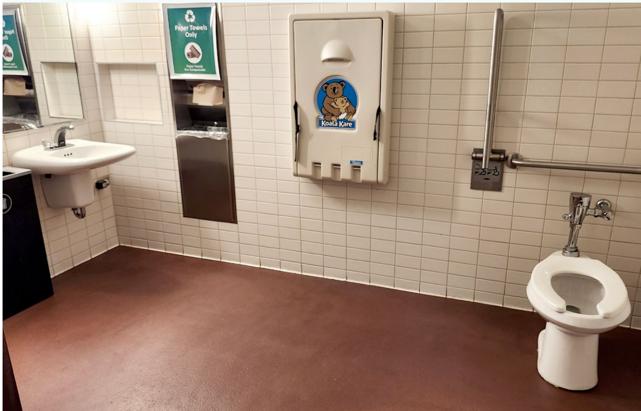
Image Description: Inside the accessible washroom. The adult changing table is not shown in this photo.
